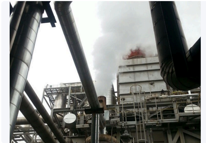
Before: flash steam venting above the condensate drum.
